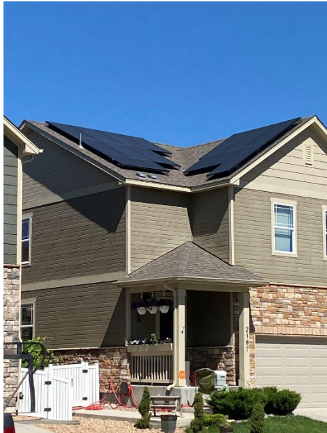
Rooftop PV System
