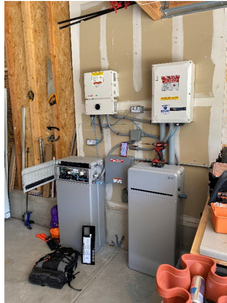
Battery Energy Storage System
