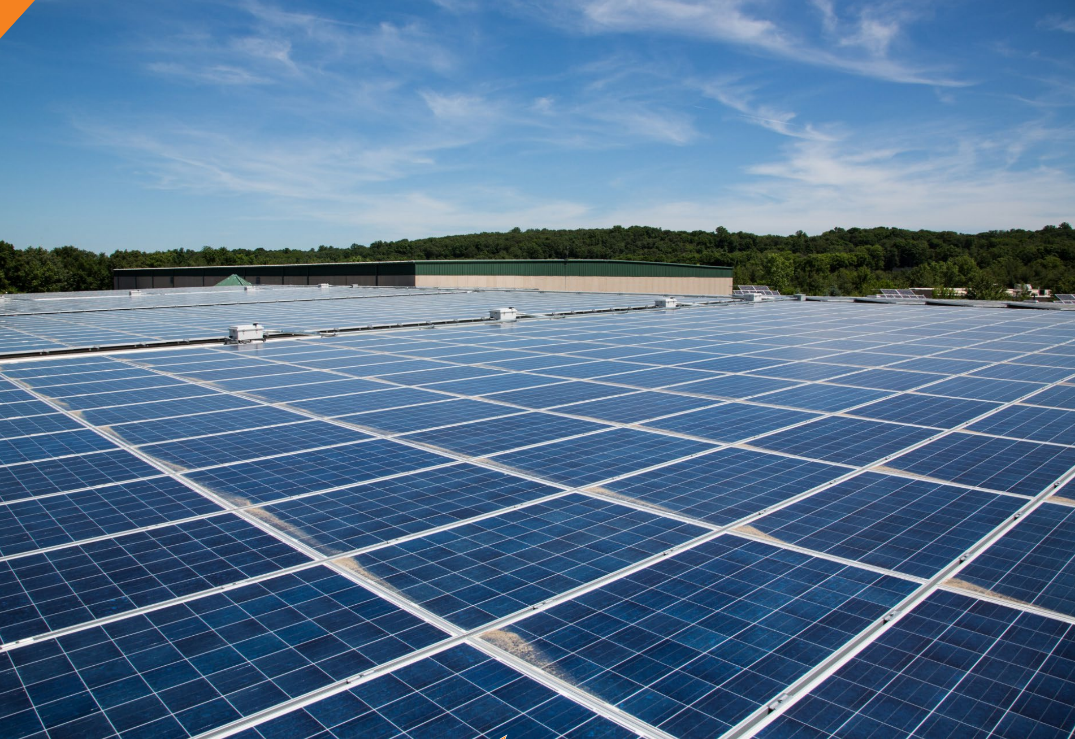
InSports Center, Trumbull, CT: Energy Upgrade to a 252 kW solar photovoltaic system; energy efficient lighting
