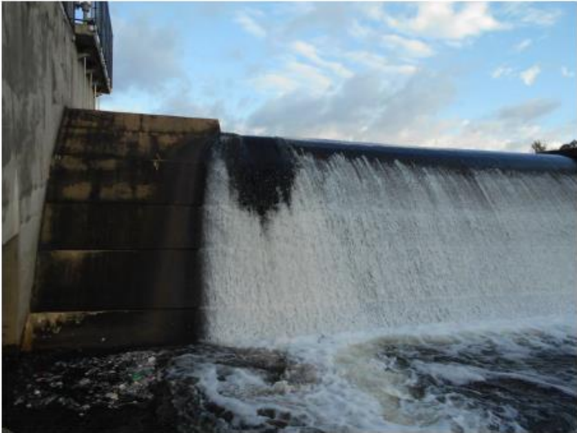
No. 3 Ogee spillway 60 feet long (Spillway No. 1) at the right training wall.
