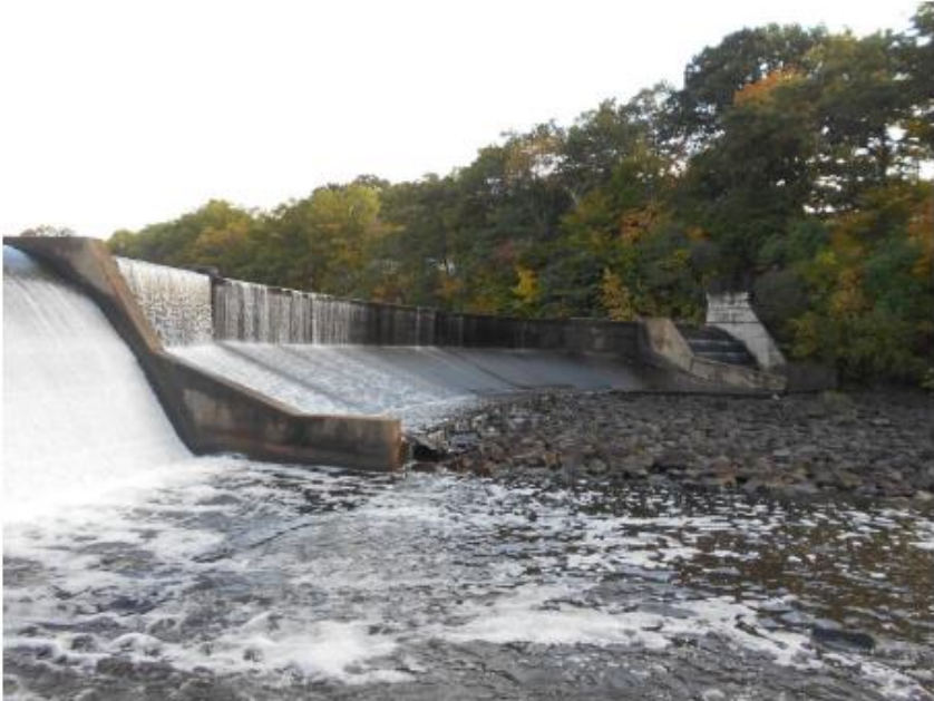
No. 4 Looking from the right at the broadcrested concrete weir center spillway section (Spillway No. 2) 147 feet in length.
