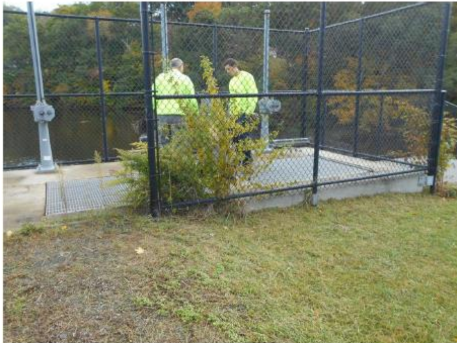
No. 8 Sluice gate operators at the inlet/outlet structure at the right training wall.
