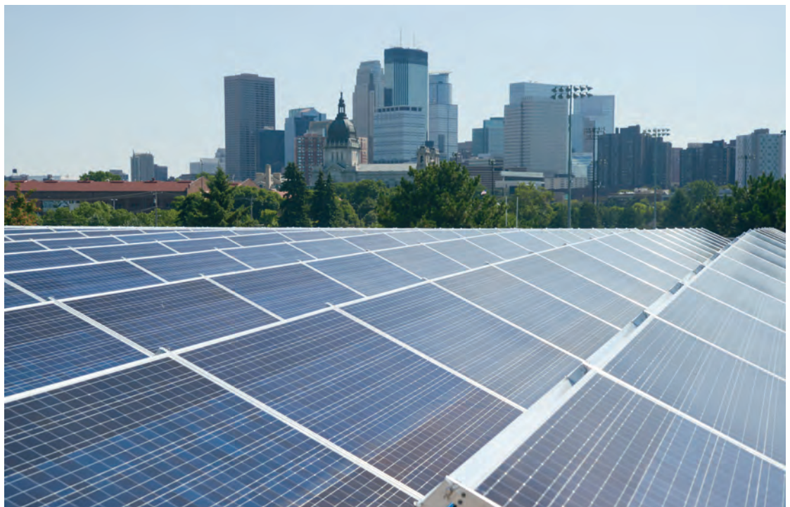
A 153-kW roof-mounted ballasted solar helps power the largest indoor ice arena in Minneapolis. Source: Minneapolis Park and Recreation Board.
