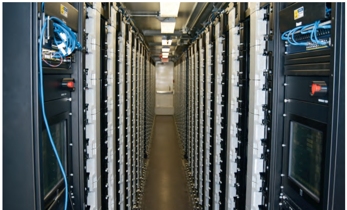
Interior of battery storage system container in Sterling, MA. Source: CESA.
