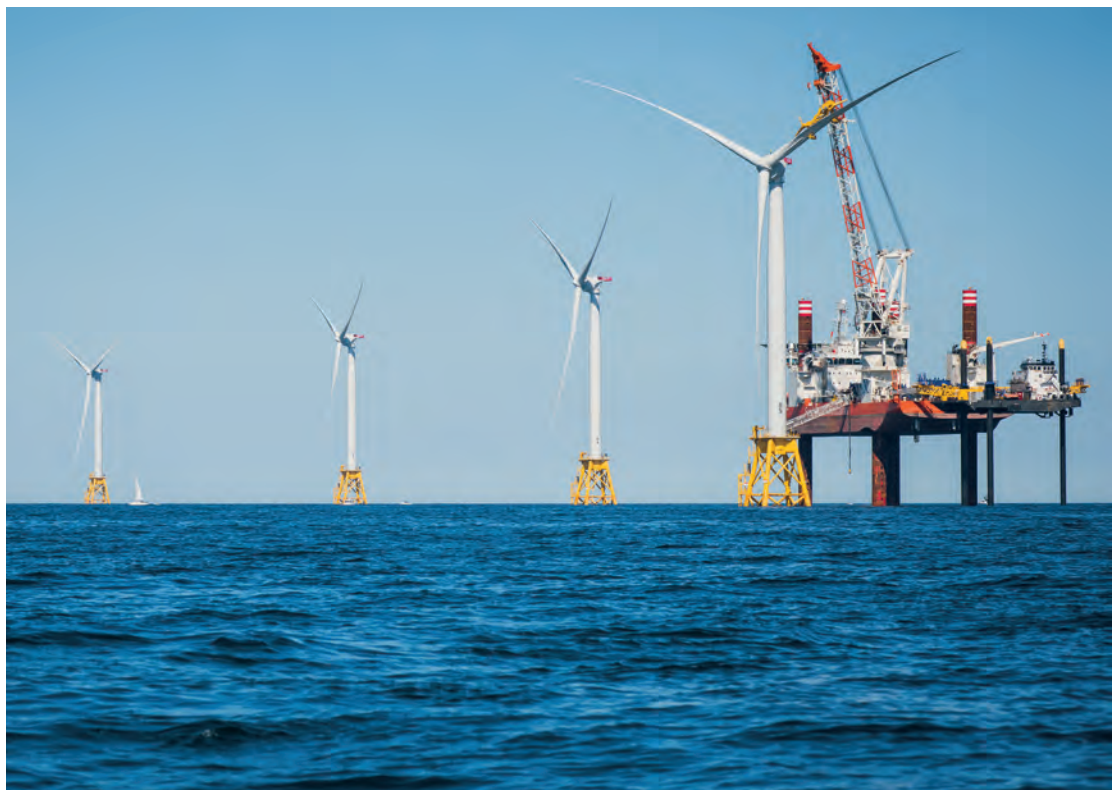
The fifth of five wind turbines being installed off Block Island, RI. Source: Deepwater Wind
