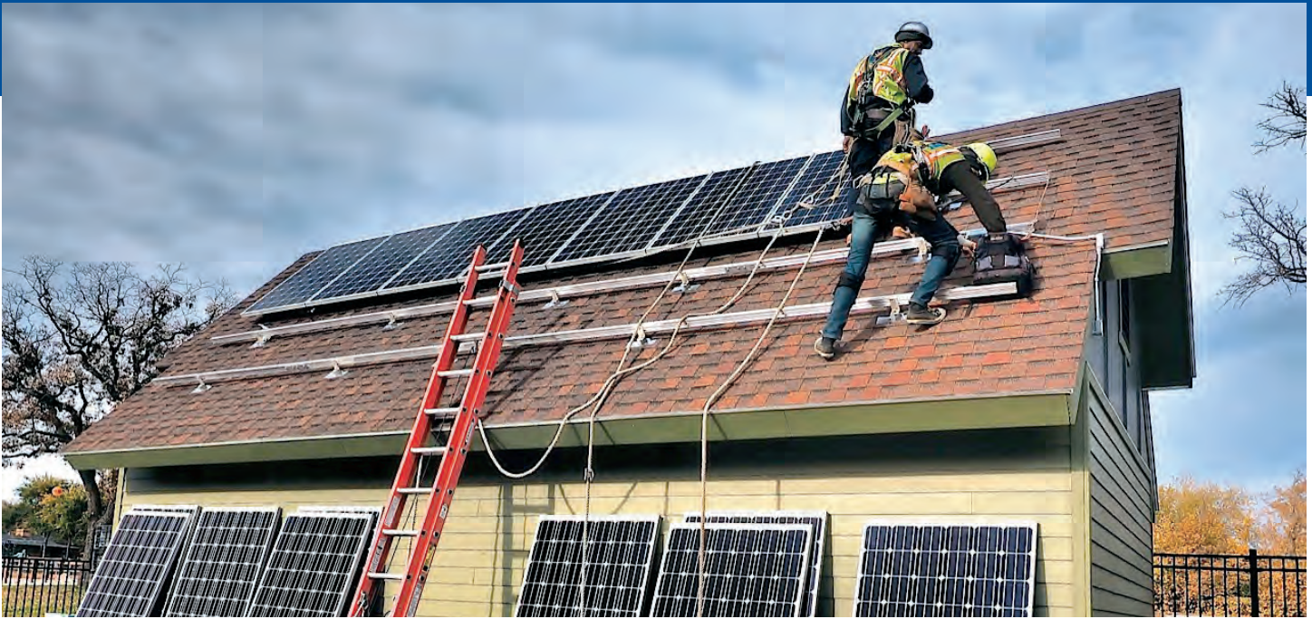
Solar installers working on the 6.4-kWh roof-mounted PV array that will power the pumps that clean the water at the Webber Natural Swimming Pool. Source: Ray Colby/Sundial Solar.
