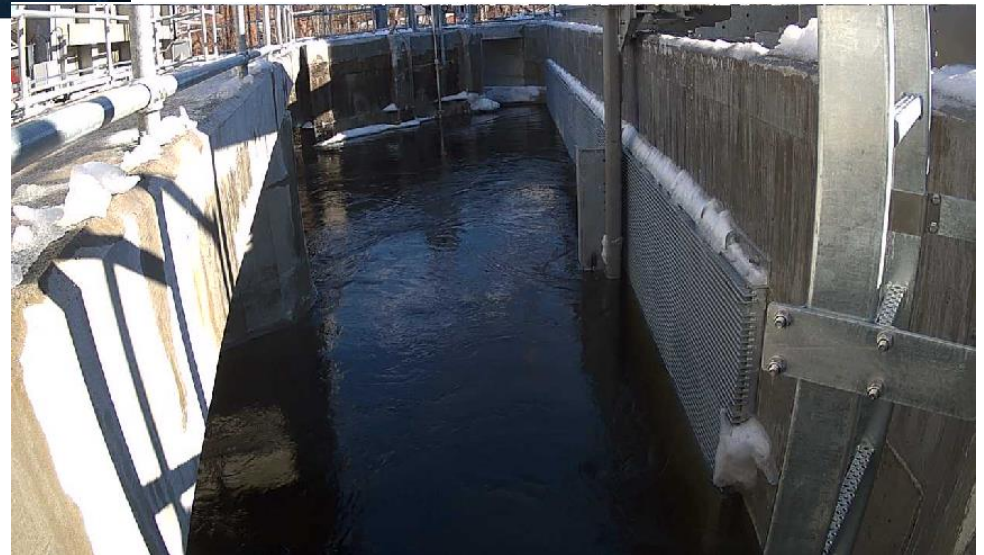
Trash rack cleaner
