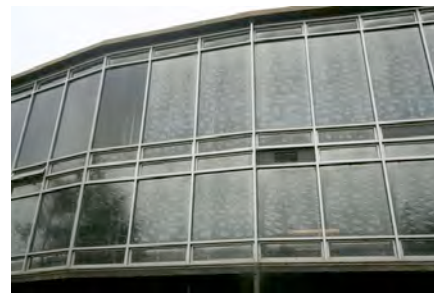
Failed window film treatment.
