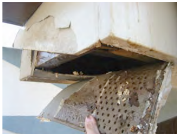
Building envelope moisture entry [Aldous 2008]
