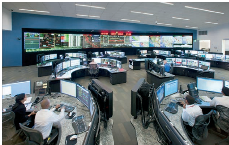
The CAISO control room utilizes synchrophasor data to manage the electric grid. Source: CAISO
