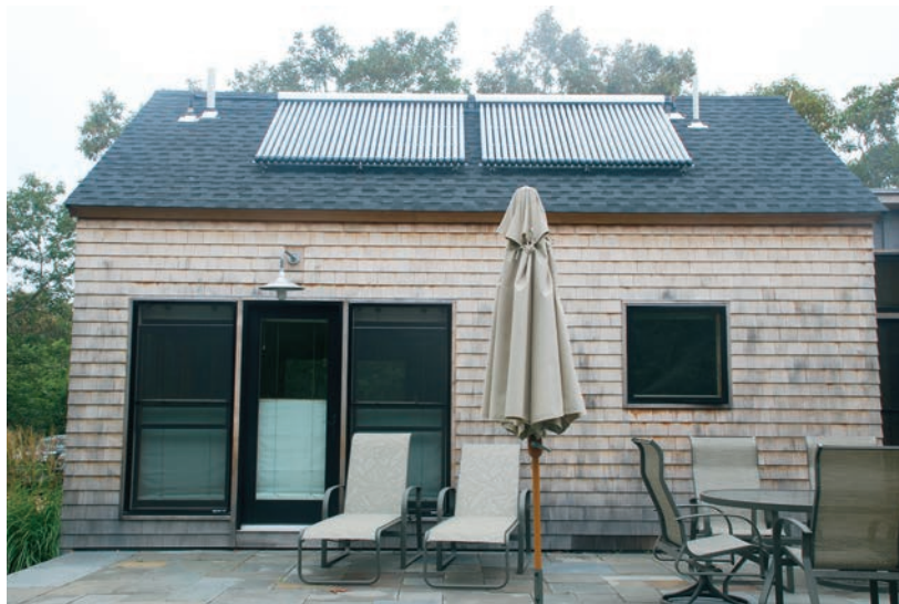
Residential evacuated tube solar domestic water and space heating system on Martha's Vineyard, Massachusetts.
