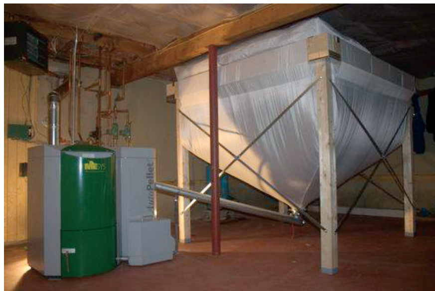
A typical storage bin and wood-pellet boiler. A bin is usually about 6' X 6', about the size of an old coal bin.
