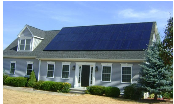
Solar PV System in Manchester, CT, Courtesy of Real Goods Solar
