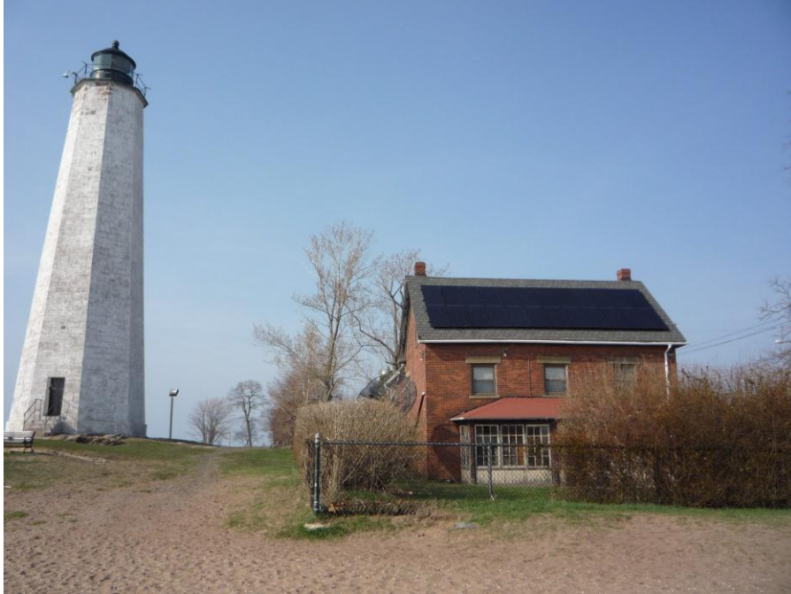
Figure 18: New Haven Lighthouse Solar PV Installation, Courtesy of Ross Solar Group
