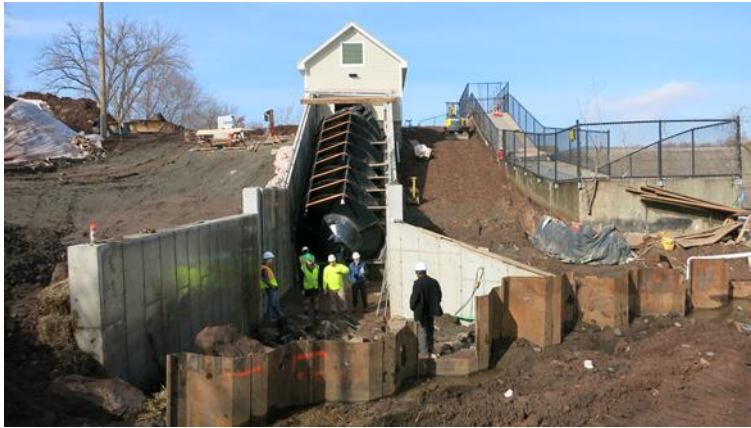
Archimedes Screw Generator installed
